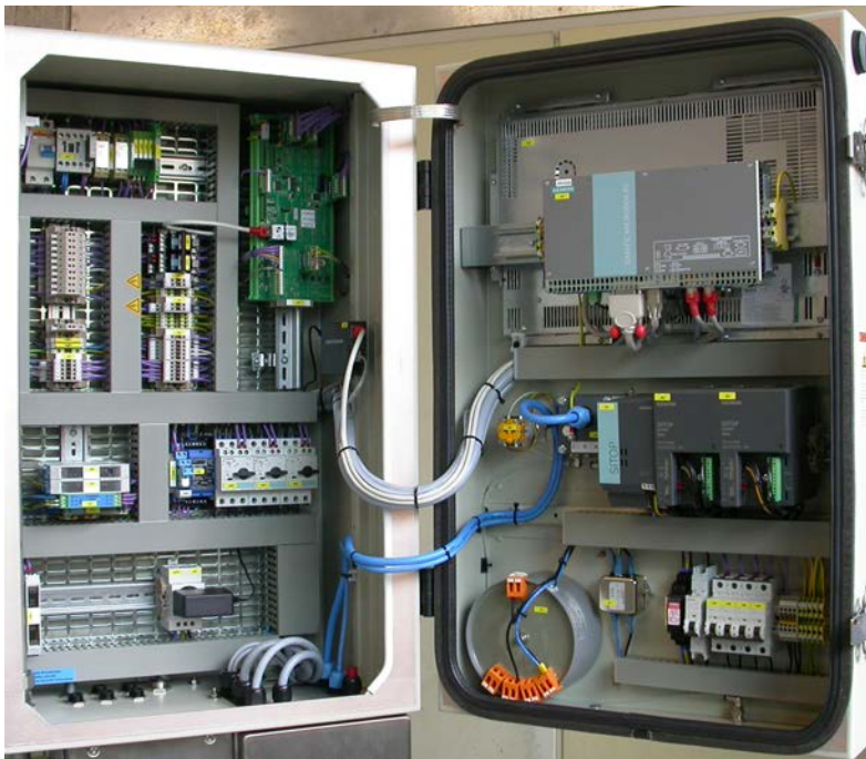
Fig. 5.5: Typical example of a control box
