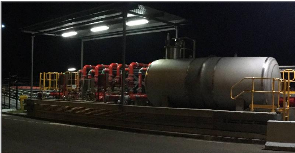
(Top Middle) A selection of foam concentrates stocked by Orion. We can supply in containers from 20L through to 1,000L IBC's. (Top Right) A 4,500L bladder tank assembly with pneumatically operated control valves. (Bottom Right) A 20,000L atmospheric foam storage tank, with 2 x Foam pumps and a number of deluge valves.
